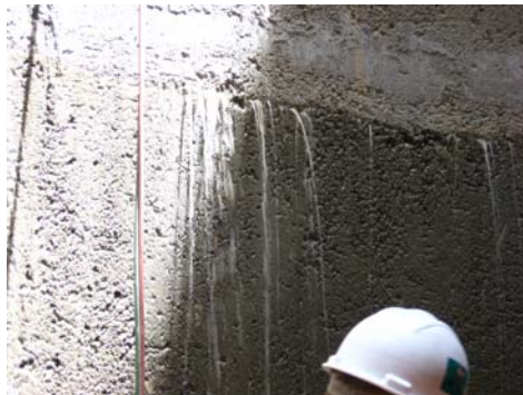
Figure 13. Water leakage through a shotcrete cold joint above the tunnel
