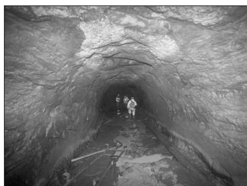
Figure 7. The first unlined tunnel also showed residual mud in the invert, which made walking difficult. Note the remnants of the one of the ladders from the intake structure.
