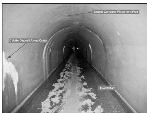
Figure 6. The portion of the tunnel above the “stored” water level lined with mud in the invert, which made walking difficult
