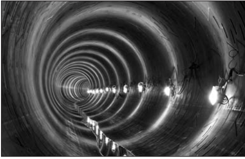
Figure 6. Use a telephoto lens to create dynamic images by compressing tunnel perspective and construction lighting. (Photo used with permission of the City of Portland Bureau of Environmental Services.)
