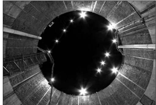
Figure 5. Use a wide-angle lens to capture dramatic overviews of underground structures, such as this night photograph of the West Side CSO Project Swan Island Pump Station Shaft. (Photo used with permission of the City of Portland Bureau of Environmental Services.)
