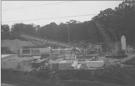
Figure 3. Top of shaft conveyor belt system
