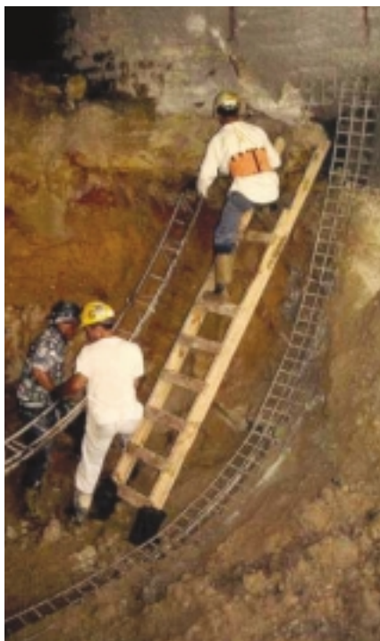
Closing the ring quickly behind the bench, as shown in this photo, is key to preventing lining instability
