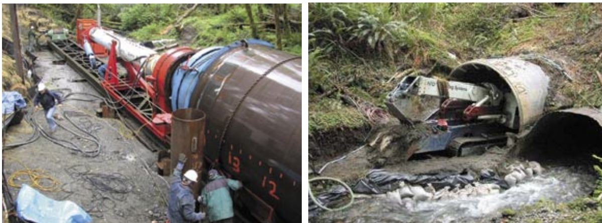
Figure 4. Pipe ramming is used to install a parallel culvert (Piehl et al., 2005): upstream (left); downstream (right).
