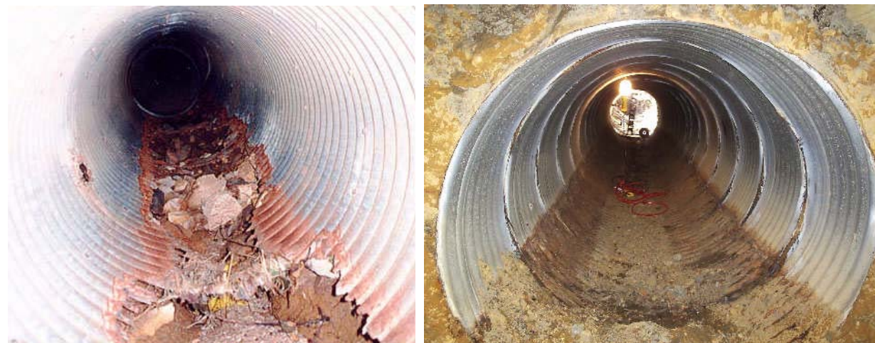
Figure 1. Typical culvert failures: corroded invert (left); squatting and splitting of the seams (right) (Tenbusch, 2009).
