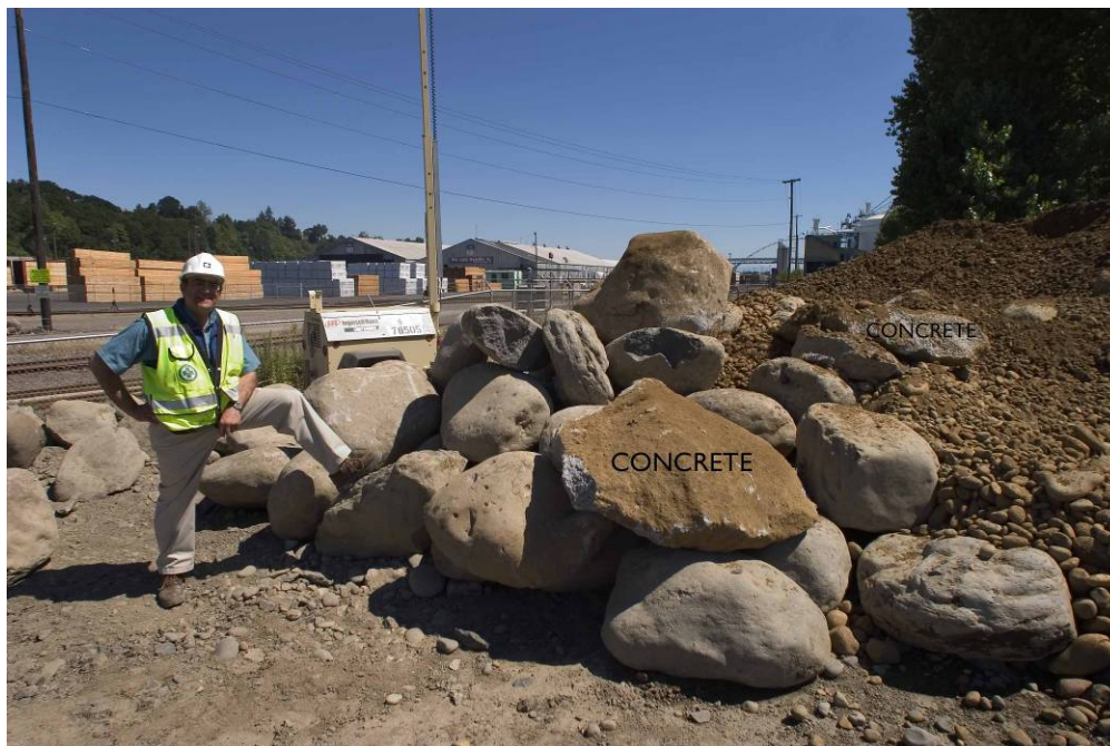
Figure 5. Catastrophic Glacial Flood boulders encountered within the Swan Island Pump Station shaft excavation (photograph by Sue Bednarz, Jacobs Associates)
