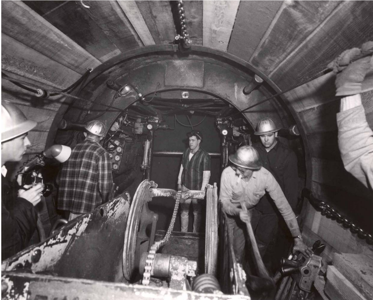
Figure 4. Workers inside the Portsmouth Tunnel shield during tunnel excavation (photo used with permission of the City of Portland Archives and Records)
