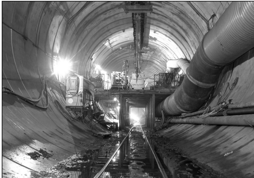
FIGURE 5. Elevated deck for construction of the adit from the Main Spine Tunnel.
